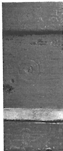
Original holes for lug.
